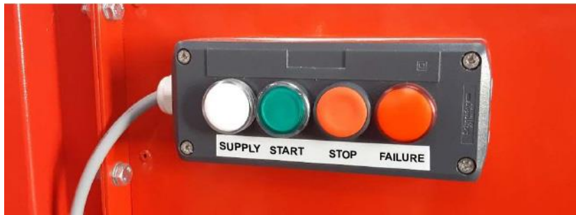
Photo No.5 – Control panel
