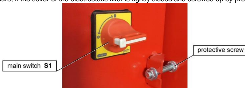
Photo No.4 – Main switch of the power supply
